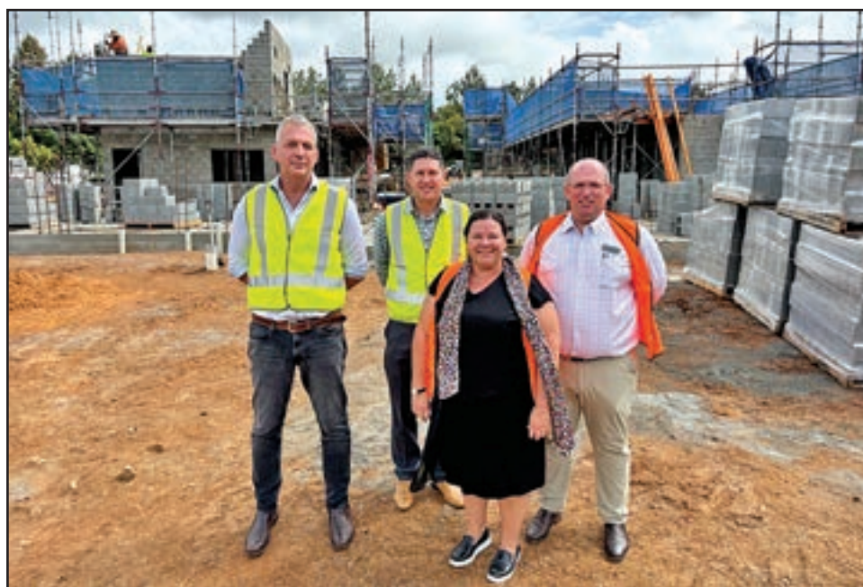
On site to see the construction progress at Djarragun College firsthand were project partners: l-r Matthew Salmon, Taro Morrison, Fiona Jose and Michael Barton.
