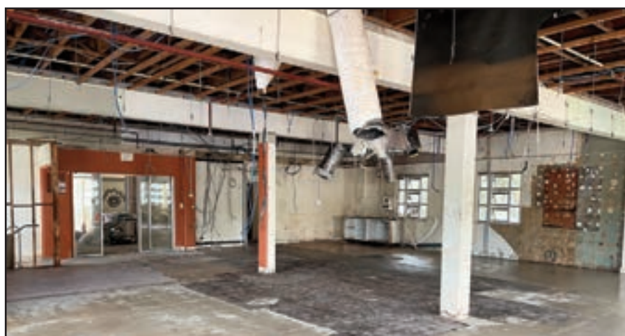
The entire first floor of the Koori Mail was submerged in the floodwaters, where up to seven offices once stood — now just a bare shell waiting on the rebuild.
